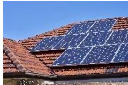
Gambar 4. 7 Solar Panel Sumber: google.com
